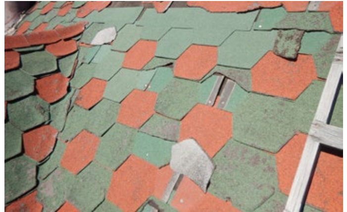
Damaged shingles on Stone House roof.
