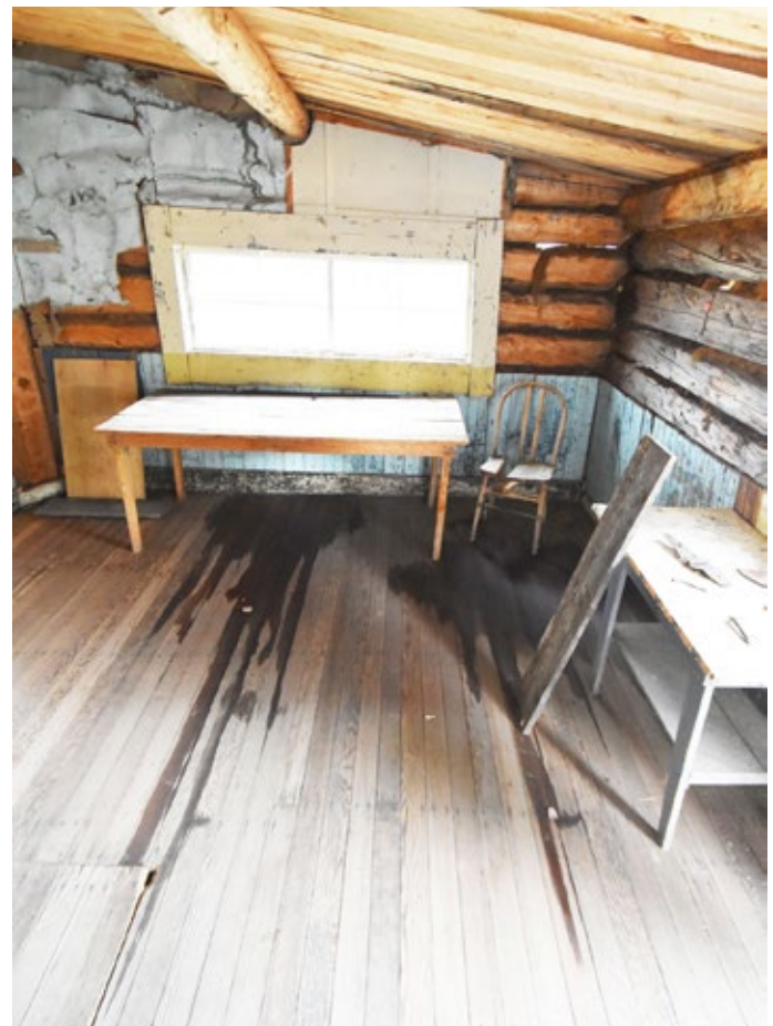
Water stains on the shed addition floor.
