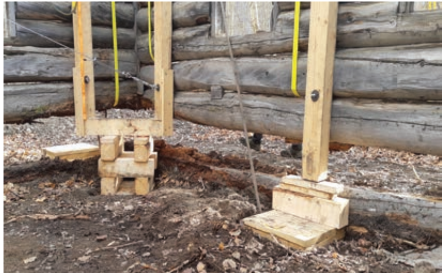
Approximately 18" lift on the highest corner.
