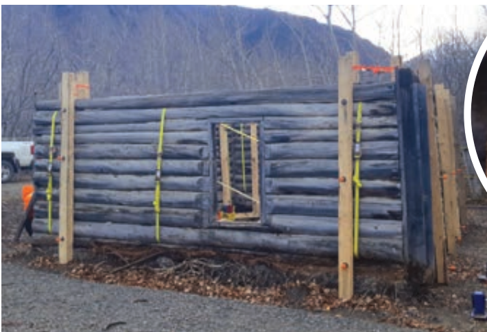
NW corner looking south prior to the lifting process, getting ready to place the jacks. Sandwich bracing is in place.
