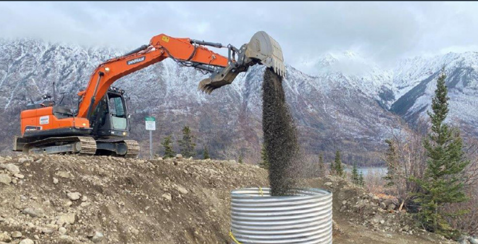
▲ Photo credit: Michael Soto. Transportation Engineering Branch. Culvert installation at Big Thing Creek. October 2021.
